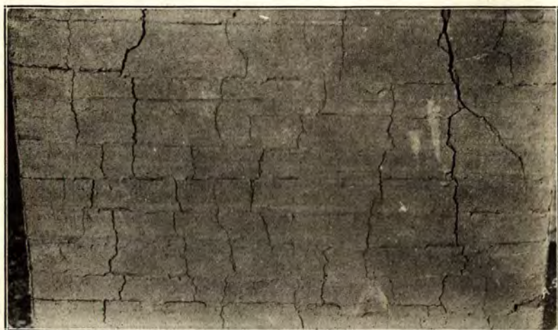
Figure 10.—A PISE WALL FROM SOIL IN WHICH THERE WAS NOT ENOUGH SAND.
